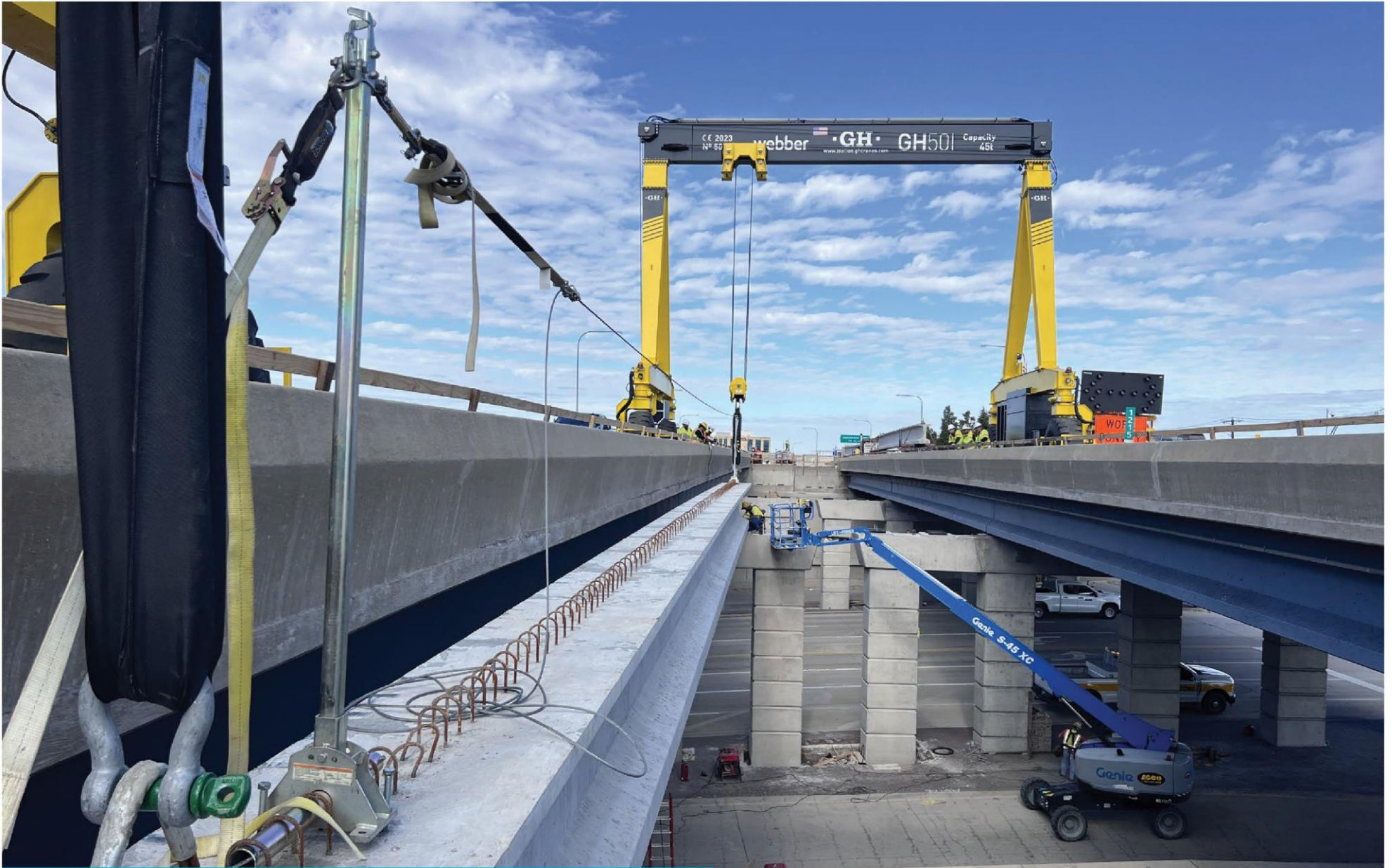
Using a gantry crane to place beams on the Dallas North Tollway Widening Project in Frisco
