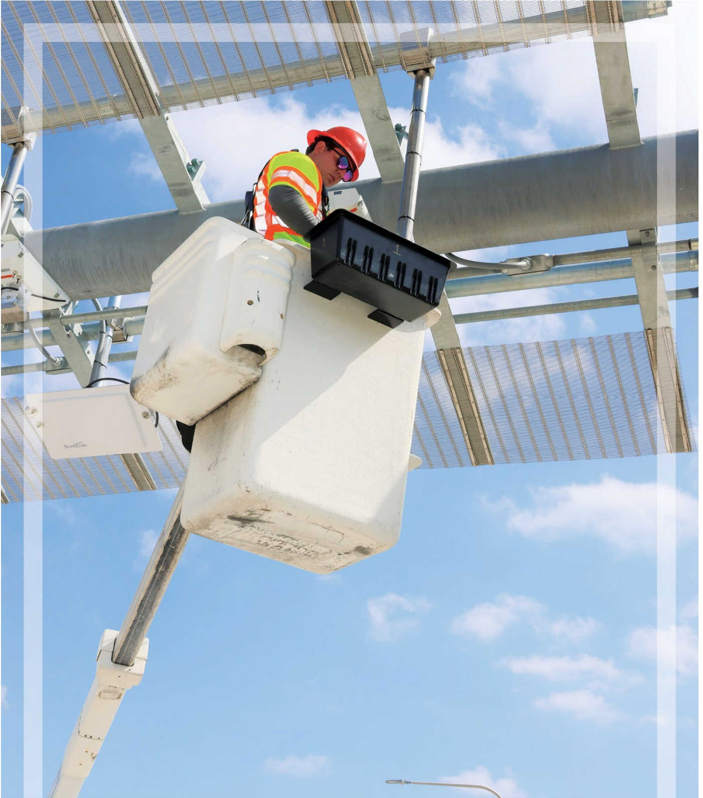
Roadway Information Technology installing new cameras at Dallas North Tollway extension bridge over US 380
