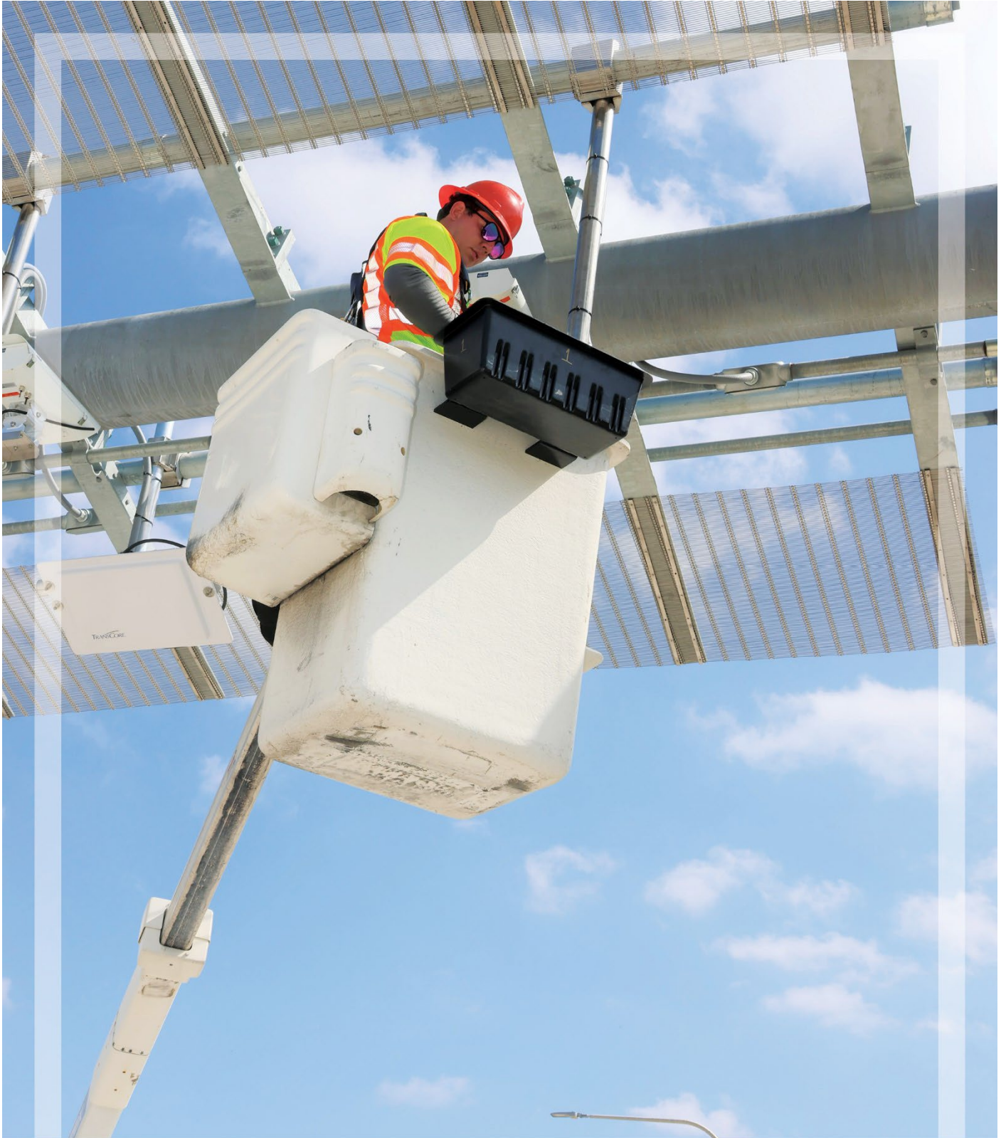
Roadway Information Technology installing new cameras at Dallas North Tollway extension bridge over US 380
