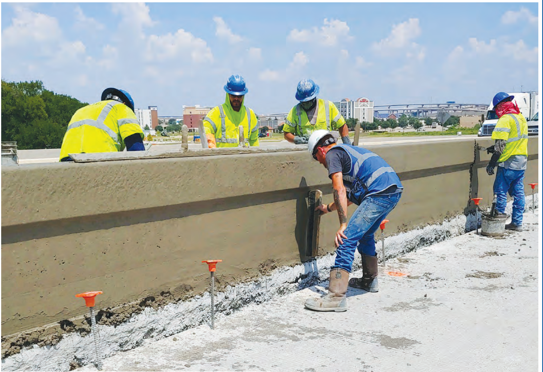
Crews perform finishing work on concrete traffic rails for the Sam Rayburn Tollway widening project
