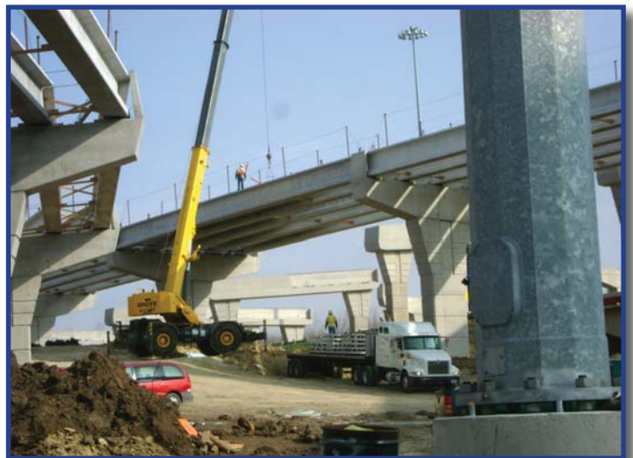
Installation of form work for bridge deck at I-20 for the PGBT Western Extension.
