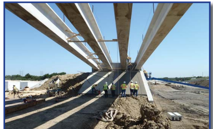
On the PGBT Western Extension project, crews inspect beams for the direct-connecting bridge to I-30.
