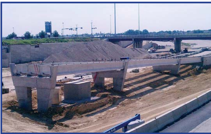
On the PGBT Eastern Extension project, bridge supports and beams are set for the SH 78 ramp in Garland.
