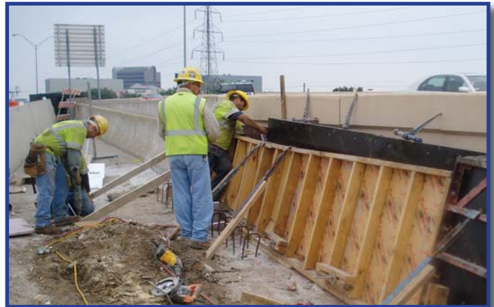
All-ETC work continued on the DNT, where crews set forms for a concrete barrier at the Spring Valley Road exit ramp.
