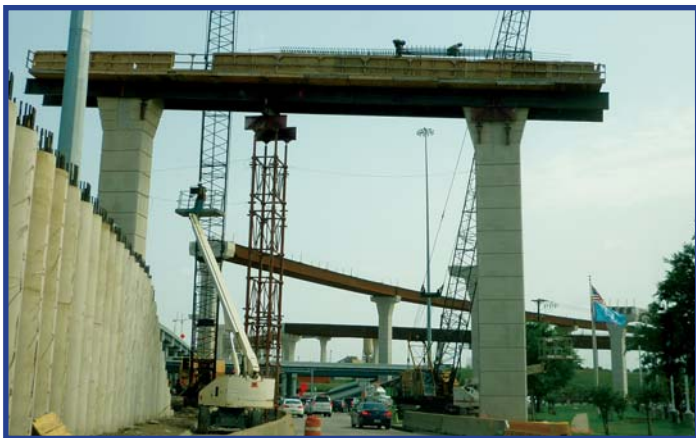
Crews work on a future bridge support that spans the southbound DNT frontage road at the SRT/DNT interchange in Frisco and Plano.
