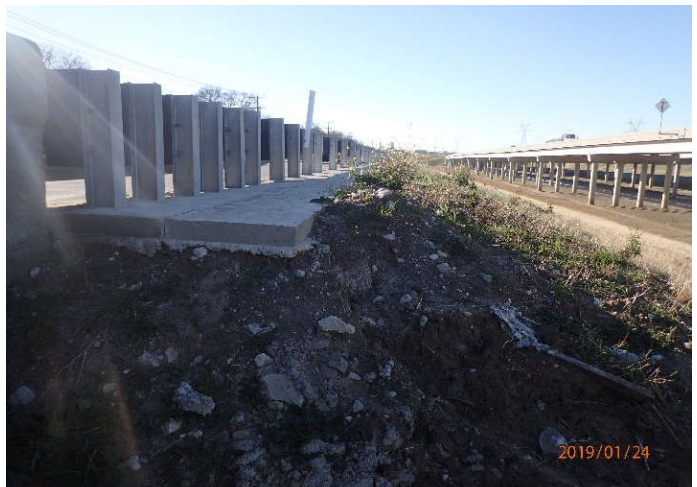
Figure 3: Erosion at Mow Strip at Walnut Creek Bridge
