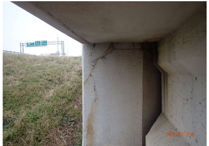
Figure 8: Backwall Cracking NB at Green Oaks
