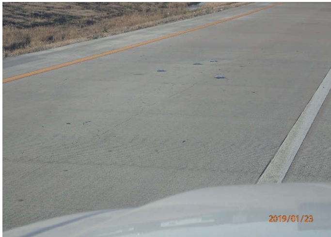
Figure 5: Missing Pavement Graphic (Arrow) SBFR at Broad Street
