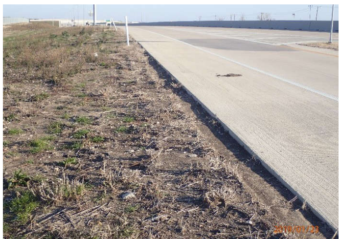
Figure 4: Pavement Edge Drop-Off at SB Ramp to Holland Road
