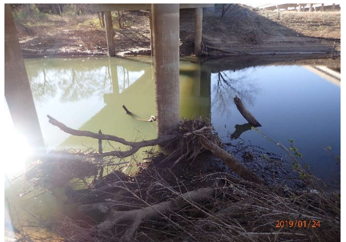
Figure 9: Debris Against Column at Walnut Creek Bridge
