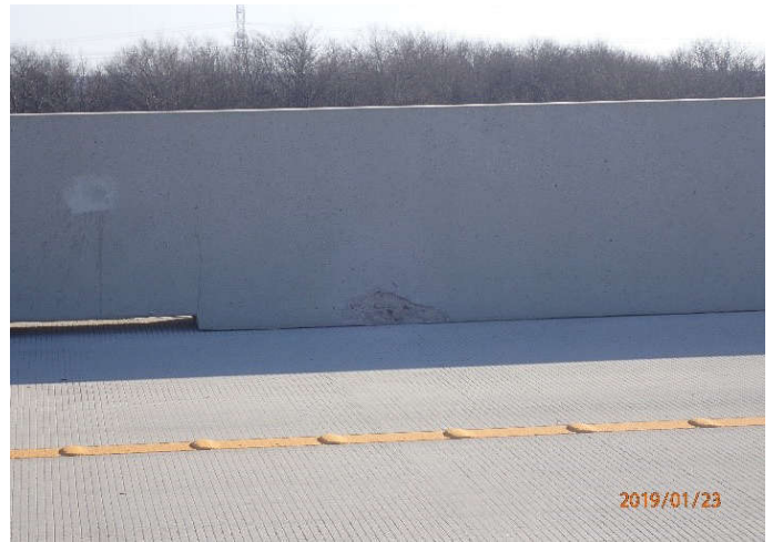
Figure 2: Barrier Rail Spall at SB 360 South of Tarrant County Line
