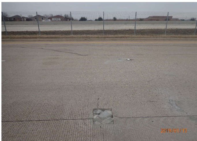
Figure 6: Pavement Spall at Rock Hill Bridge
