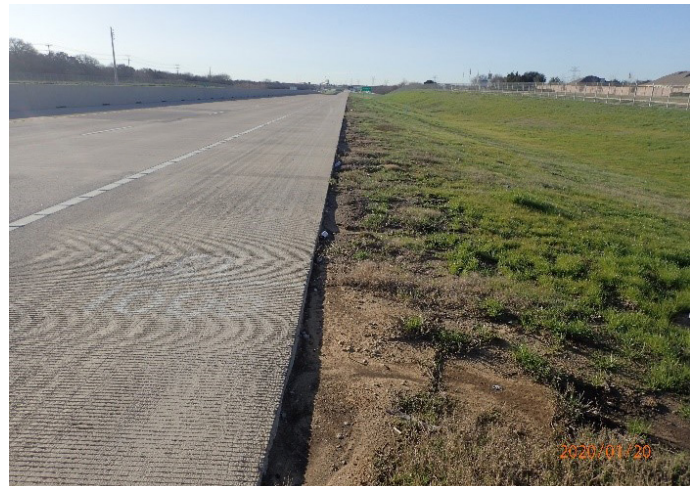
Figure 2: Pavement Edge Drop-off
