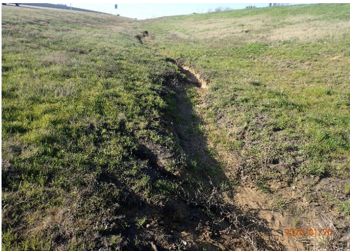
Figure 6: Ditch Line Erosion
