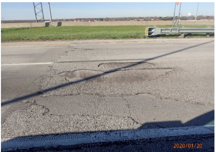
Figure 4: Asphalt Pavement Delamination
