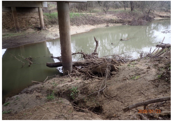
Figure 8: Debris Against Column at Walnut Creek Bridge
