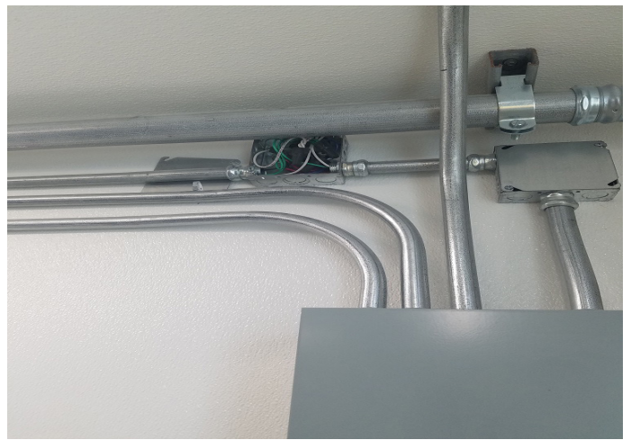
Figure 9: Cover Missing on Junction Box
