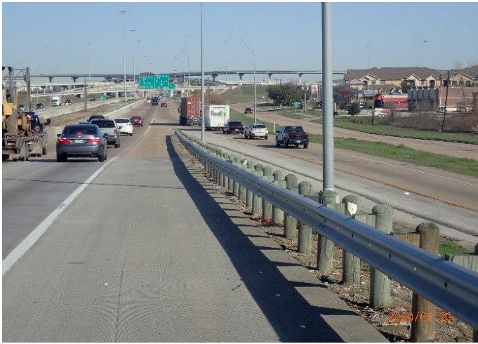
Figure 5: Delineation Missing on Guardrail
