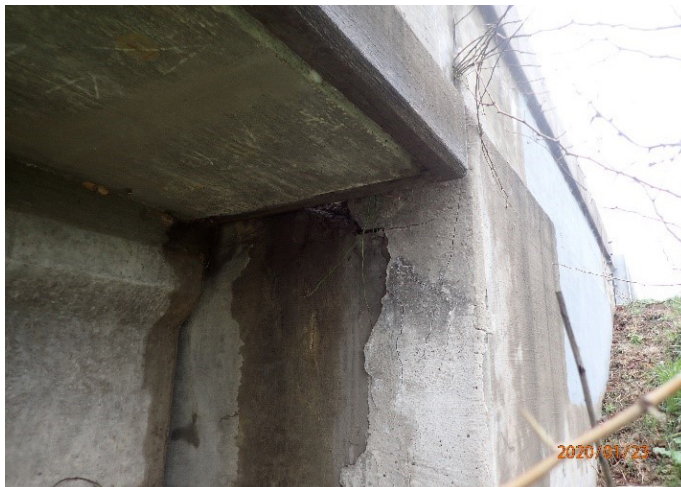
Figure 7: Backwall Cracking at Walnut Creek Bridge
