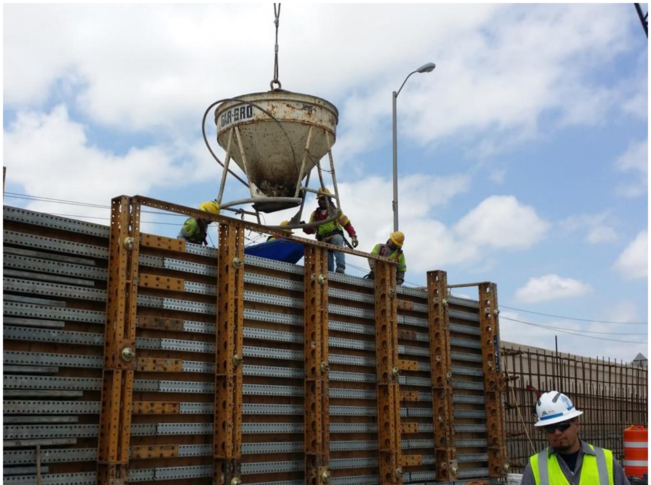
Pouring the new cast in place wall along the southbound main lanes
