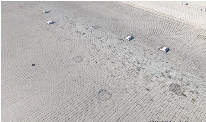
Figure 8: Reflective Pavement Markers Missing at Exit Ramp Sta. 787+00
