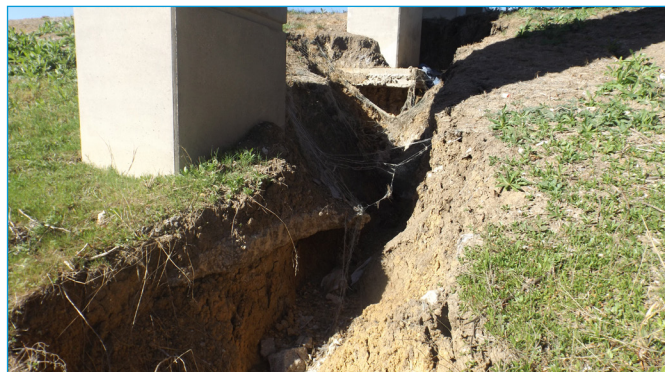
Figure 3: Erosion along Frontage Road Bridge Columns Sta. 125+00
