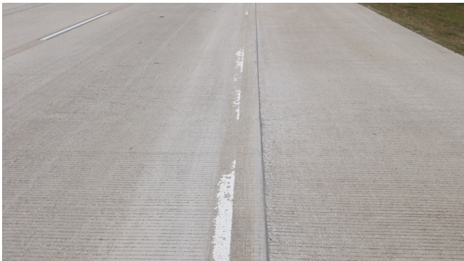
Figure 6: Faded Pavement Markings on ML Sta. 445+00
