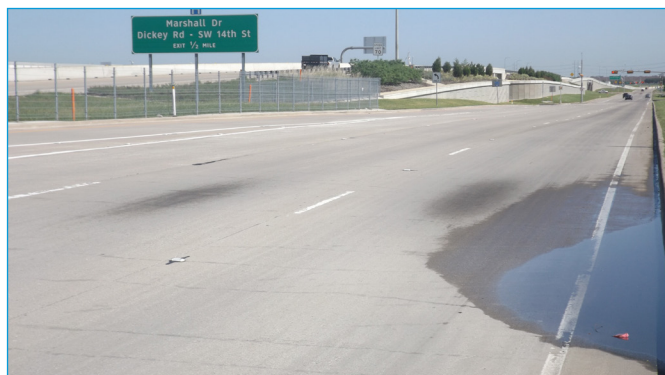
Figure 4: Frontage Road Settlement SB Sta. 122+00
