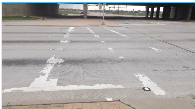
Figure 5: Faded Pavement Markings on Frontage Road at Mayfield Road
