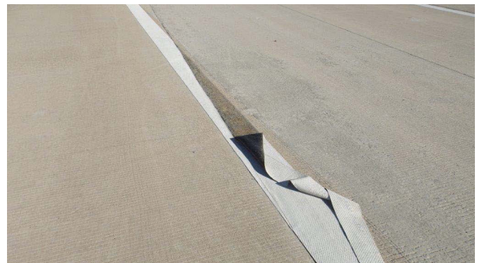
Figure 7: Pavement Markings Peeling at Entrance Ramp Sta. 1127+00
