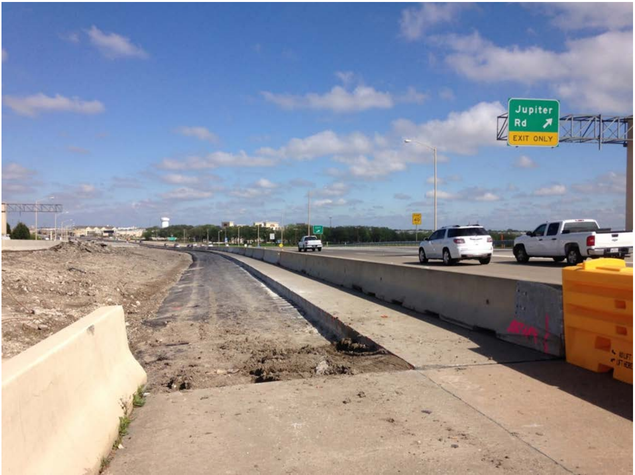
Asphalt in place for the base of the new 4 th lane westbound PGBT near Jupiter Road
