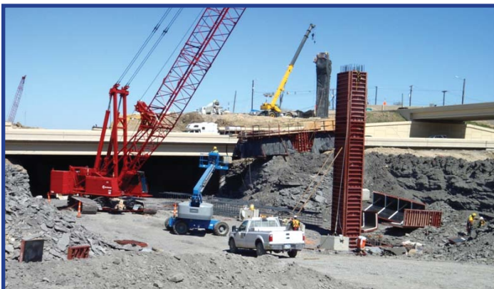
PGBT Western Extension crews work to construct columns adjacent to the I-30 main lanes.
