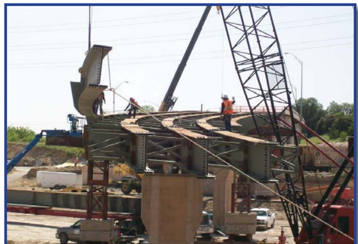
In this photo taken after only a few days of construction, CTP crews install the Rosedale Street connectors over Vickery Boulevard in Fort Worth.
