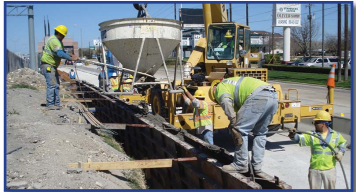
Crews pour a new concrete barrier as part of the all-ETC conversion on the DNT at Frankford Road.
