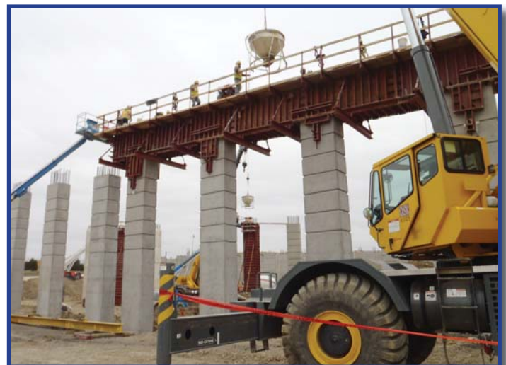
PGBT Western Extension crews pour concrete for bridge support at January Lane.
