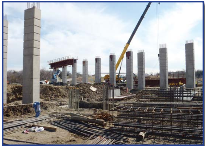
On the PGBT Western Extension project at I-30, crews work constructing bridge support at January Lane.
