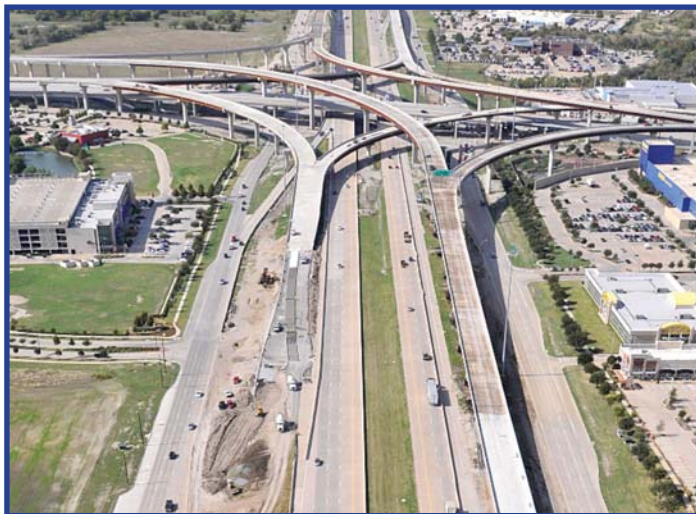
Crews are working to finish final tasks on the SRT/DNT interchange, which fully opened in mid-November 2011.
