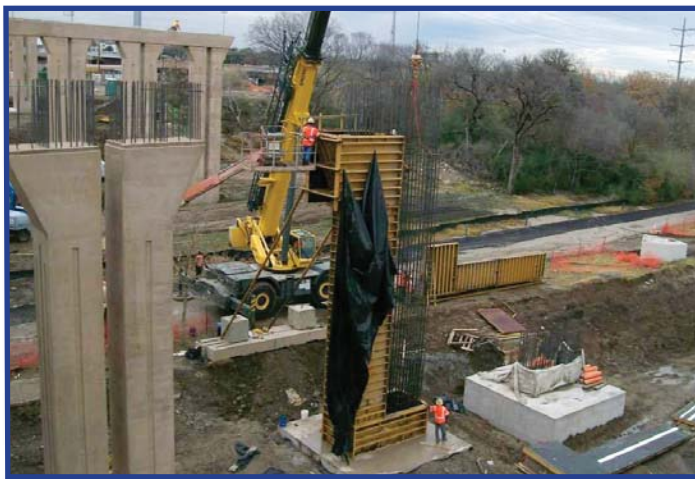
On the CTP project, crews set column forms and steel reinforcing cages for new Hulen Street bridge.
