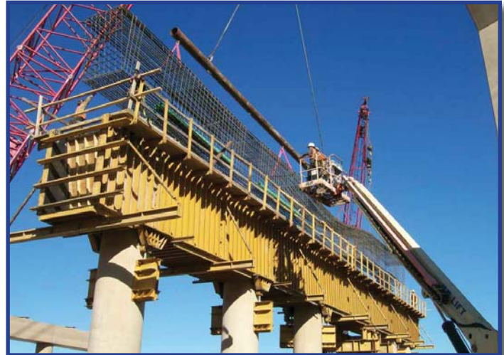
On the Chisholm Trail Parkway, crews place reinforcing steel cage for northbound main lane bridge support for the future Hulen Street bridge.
