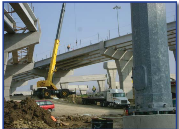
Deck panel placement for the I-20 direct connector at SH 161 for the PGBT Western Extension.
